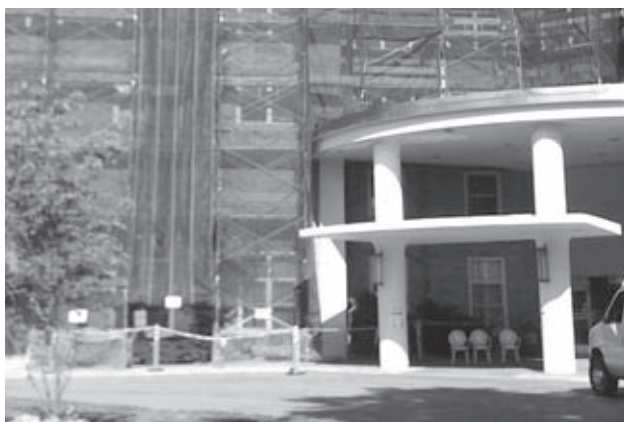
View of the front entry with scaffolding for masonry repair during the fall of 2010.
